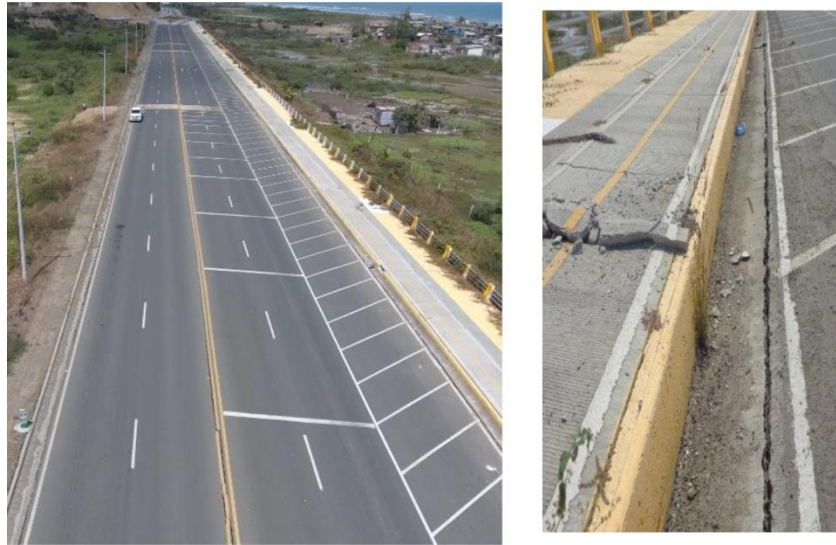
Figure 4. Minor repairable post-earthquake damage at the RAP-supported Briceño bridge embankment (courtesy of X. Vera-Grunauer)
