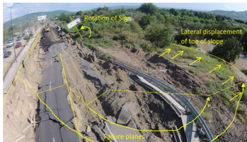
Figure 1. Mejía River Bridge Unsupported Approach Embankment (Nikolaou et al. 2016).
