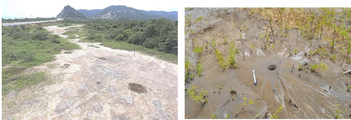
Figure 3. Sand boils indicative of liquefaction at the Boca de Briceño Bridge site (courtesy of X. Vera-Grunauer)
