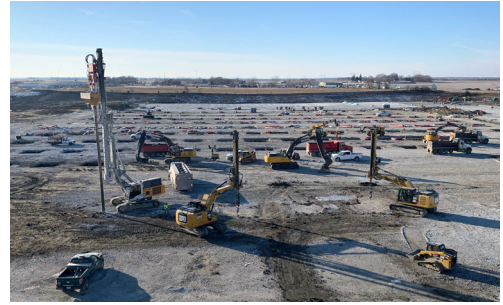
640,000 Sq. Ft. Fulfillment Center: Bondurant, Iowa 7,600 Geopier® elements piers were constructed in 48 days, shaving three weeks from the construction schedule.
